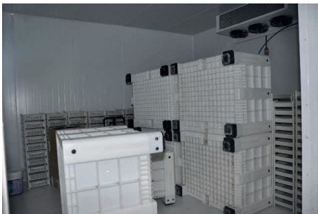
Foto 6 Fish freezing chamber
